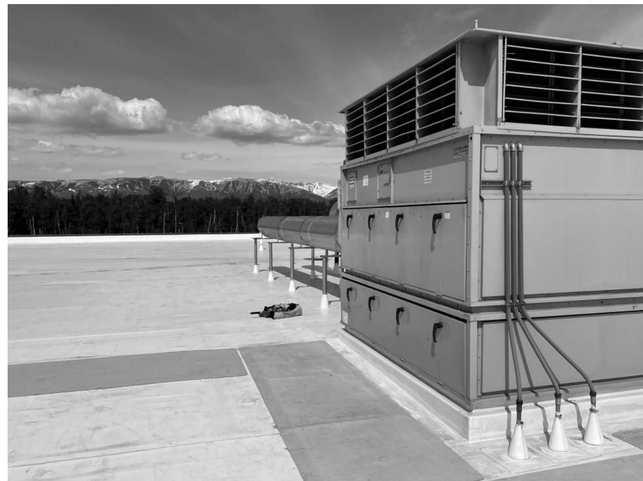
ROOF E - ERV-1
