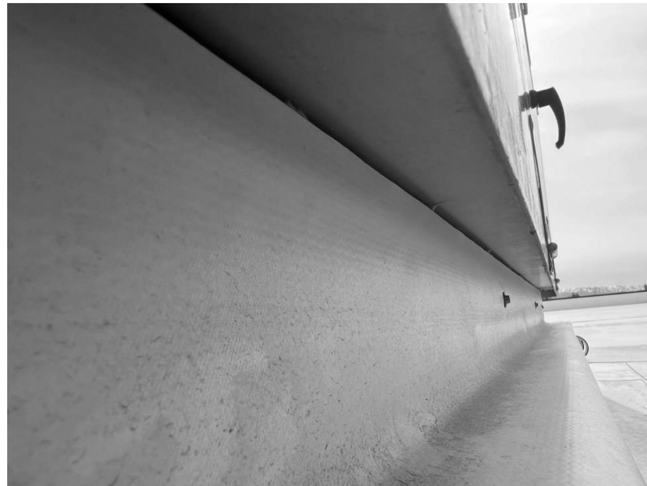
ROOF E - ERV-1 TERMINATION
