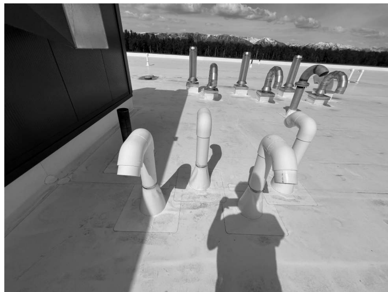
ROOF E - EXHAUST DUCTS
