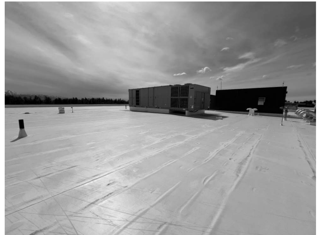
ROOF E - AHU-2
