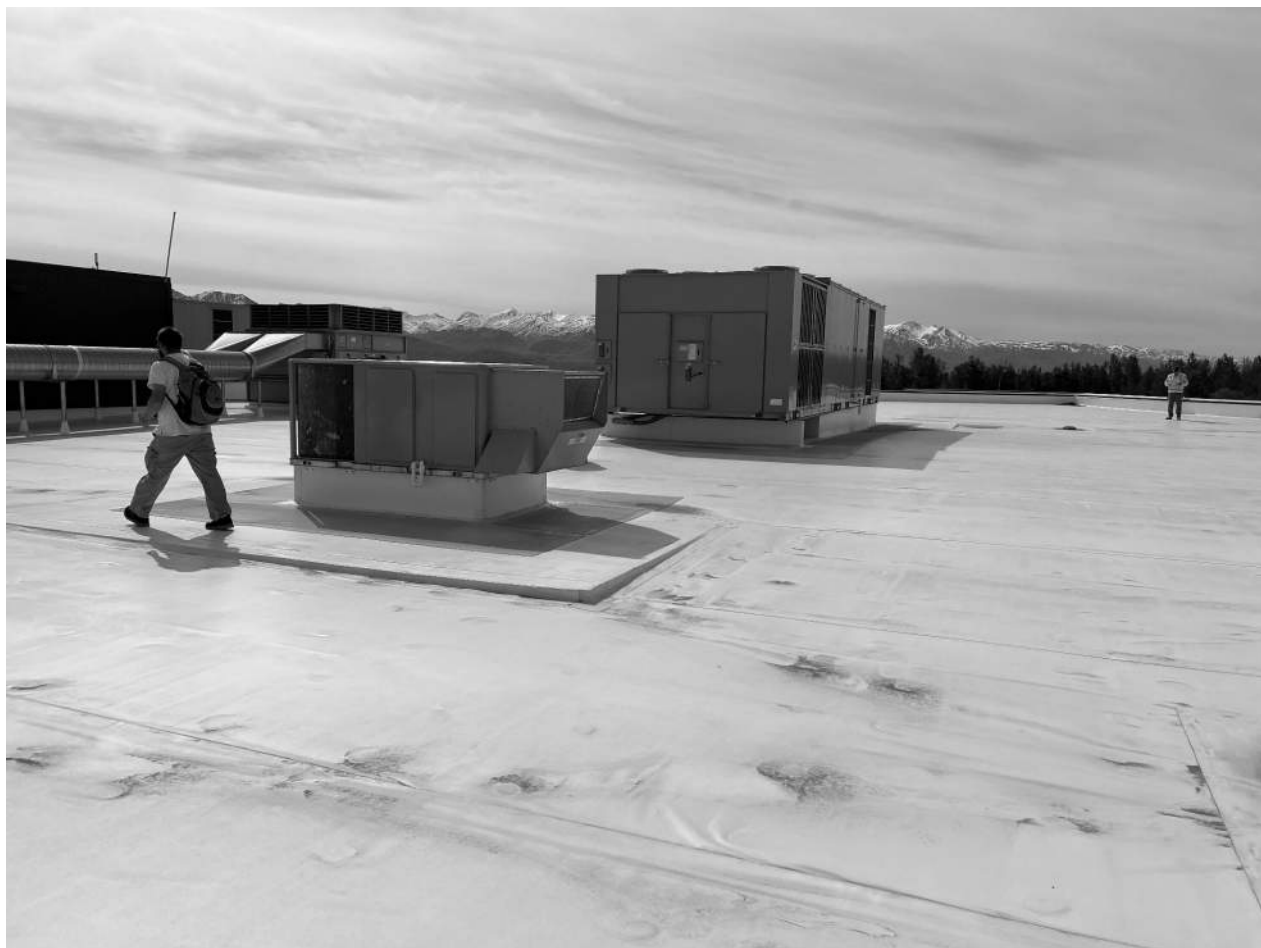
ROOF E - AHU-3
