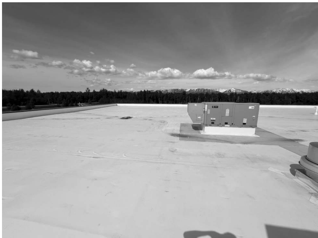
ROOF E - AHU-3
