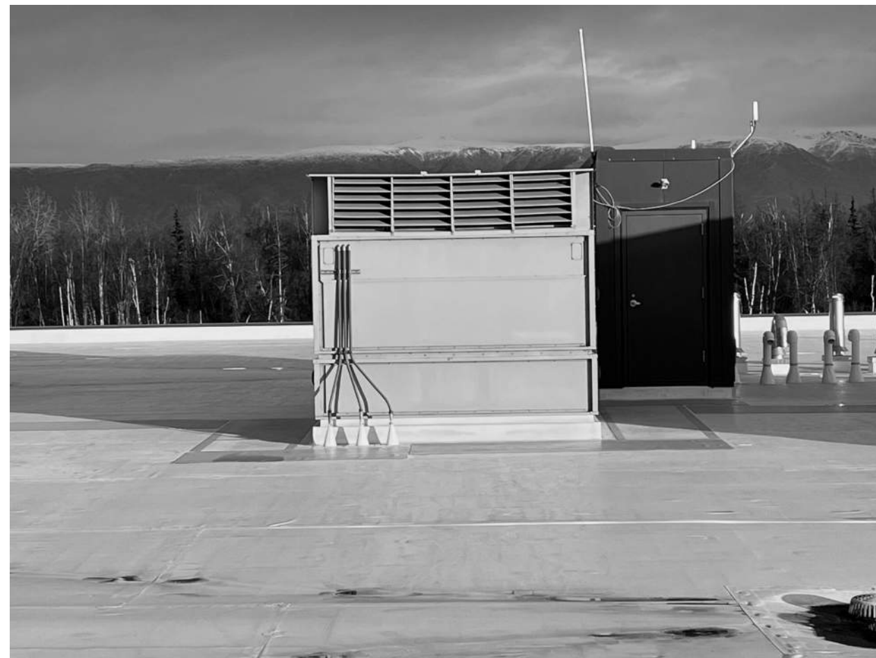
ROOF E - ERV-1
