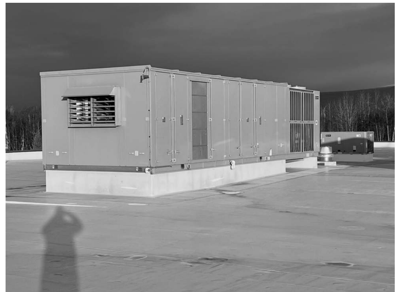
ROOF E - AHU-1
