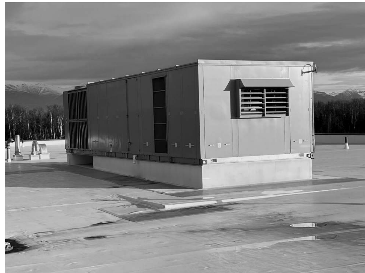
ROOF E - AHU-2
