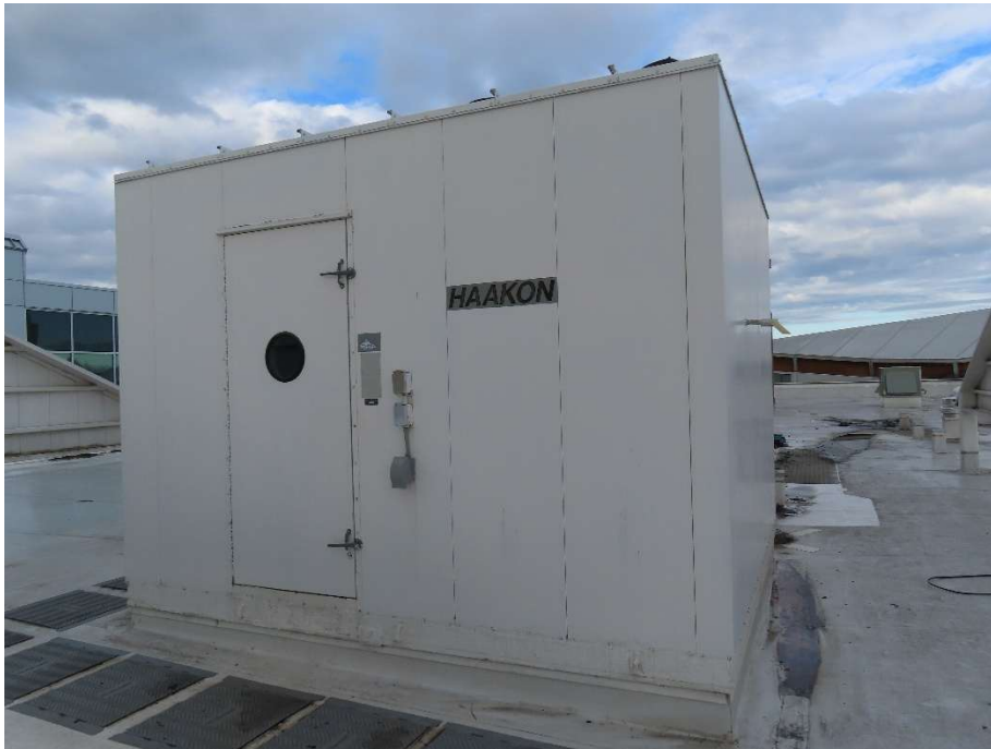
PCC1 penthouse “boiler in a box”
