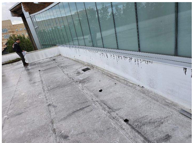
Atrium – PCC 2 sidewall condition
