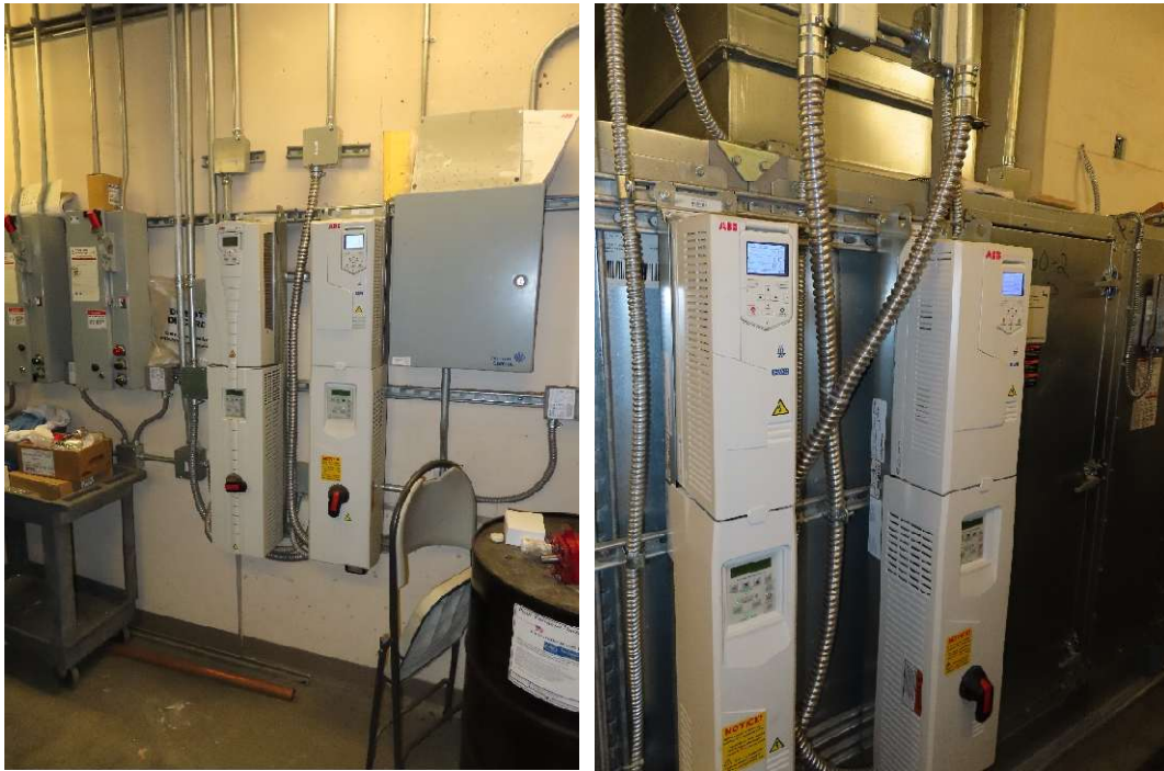
PCC3 heating circulation pump VFDs (photo at left) and AHU-3 fan motor VFDs in 2 nd floor fan room (photo at right)
