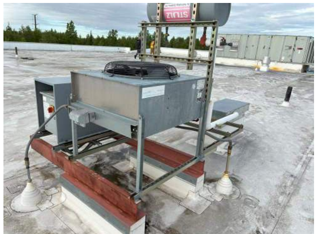
PCC 3 Roof – dry cooler
