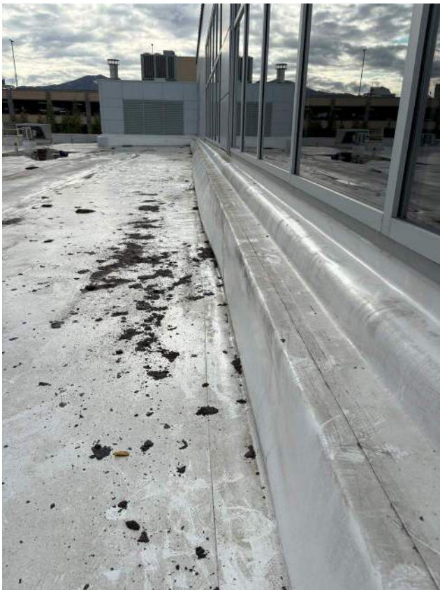
PCC 1 Roof – billowing at south sidewall
