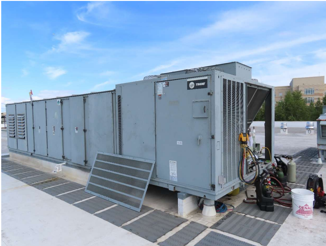
PCC2 rooftop unit RTU-B (aka RTU-2)
