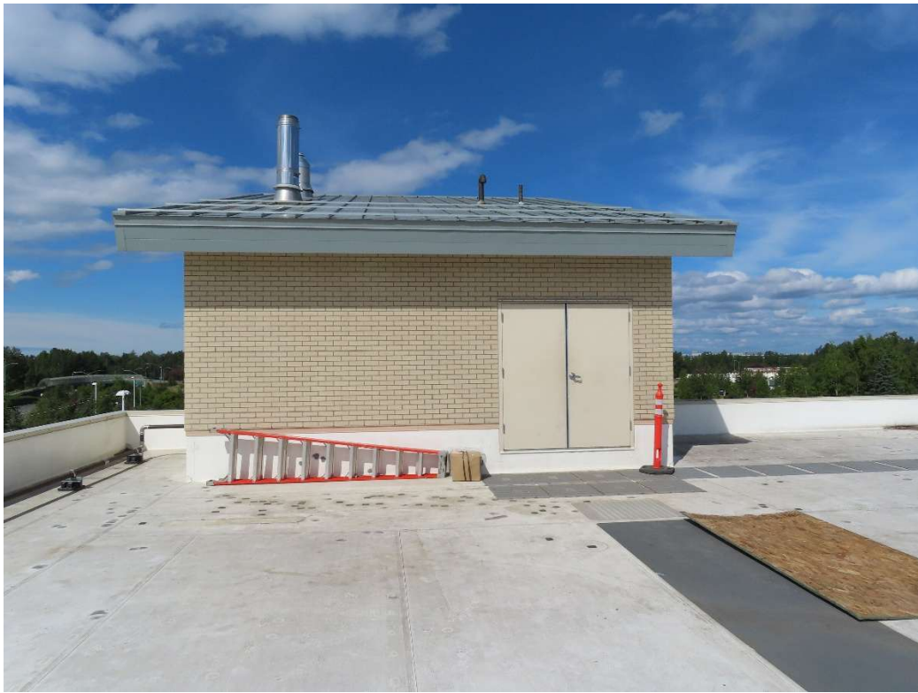
PCC2 boiler mechanical room exterior
