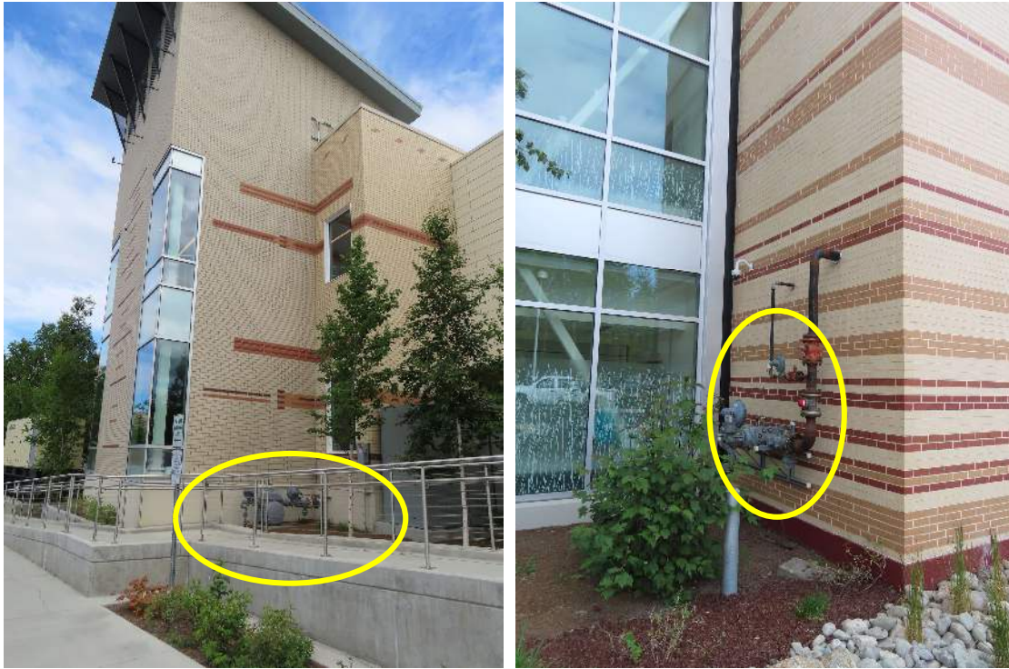
Gas meter #738 on west wall (left photo) and presumably, meter 192112 on NE corner of PCC1 (right photo), although the meter number for the NE meter do not match up with accounting invoices
