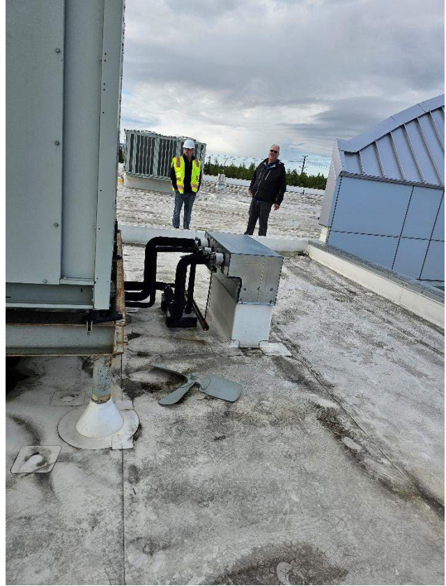
PCC 3 Roof – air handler pipe chase
