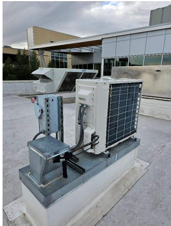
PCC 1 Roof – CU-2
