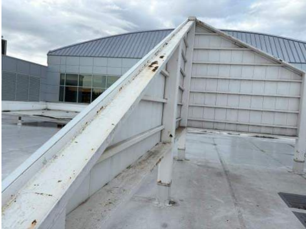
PCC 1 Roof – equipment screen
