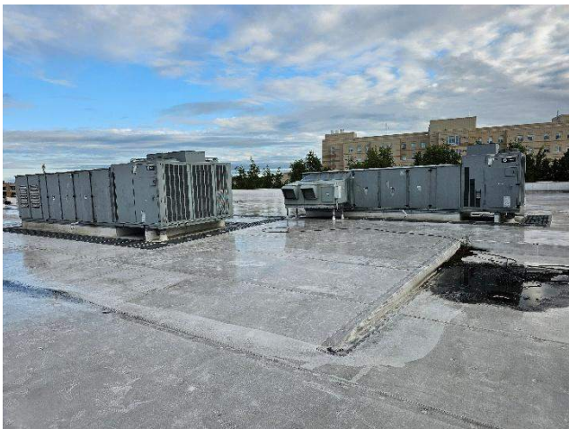
PCC 2 Roof – south side, looking north at air handlers
