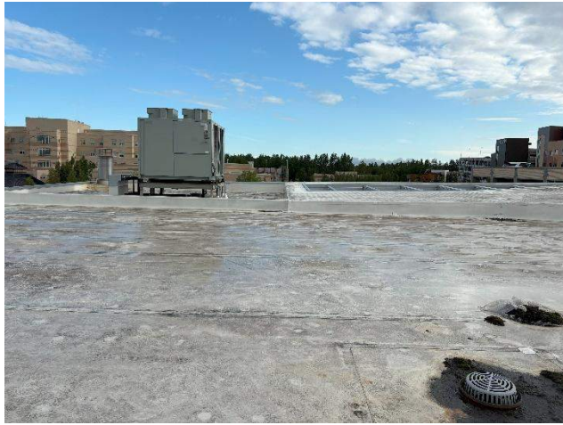
PCC 3 Roof – northeast subsection, chiller unit
