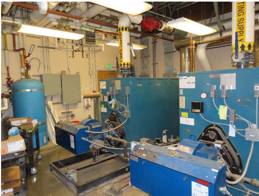
PCC3 boiler mechanical room, hot water generator shown at left, boiler re-circulation pumps above both boilers
