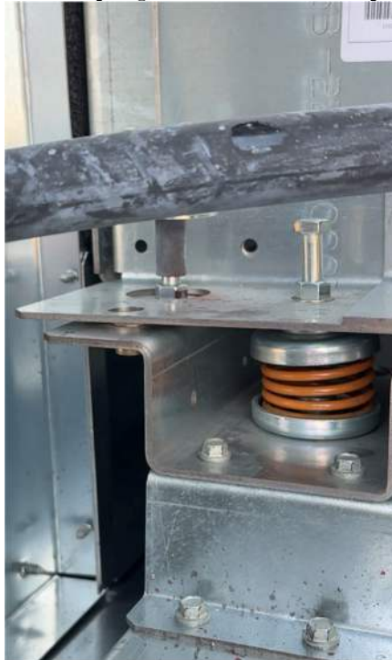
Figure 7: Bottomed out spring isolator in RTU-2.4 (potentially overloaded)
