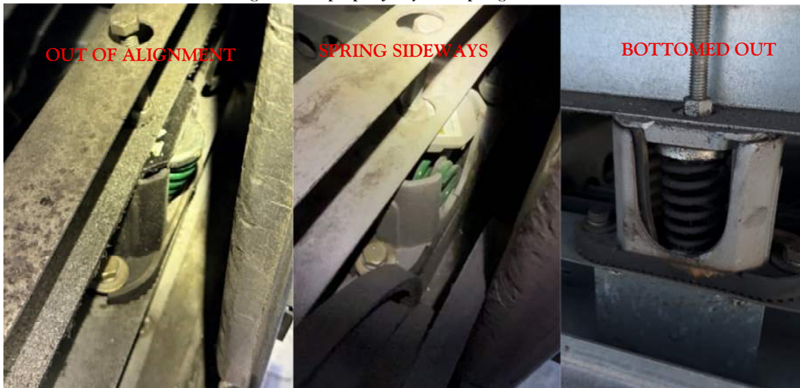
Figure 2: Improperly adjusted spring isolators
