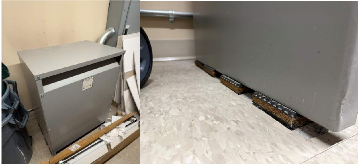
Figure 3: Electrical 2309 transformer and existing support pads
