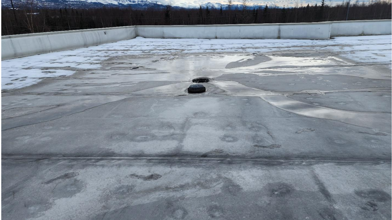
Figure 1 – Facility Condition Assessment Deficiency Photo – PCC III
