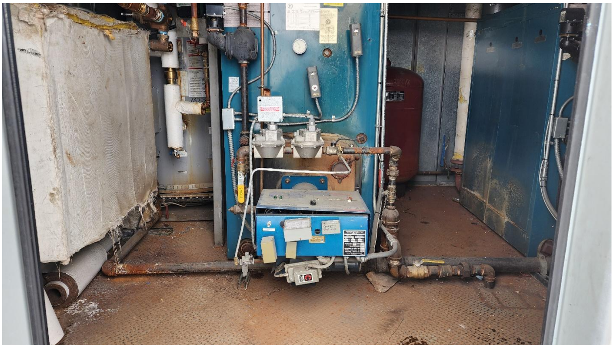
Figure 2 – Facility Condition Assessment Deficiency Photo – PCC I Boiler Room
